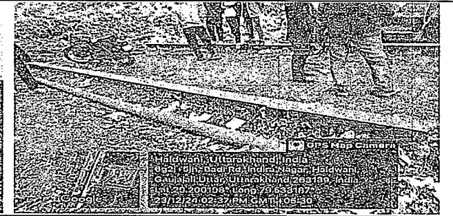
Photo 10: Weighing bridge not working at trenching ground
