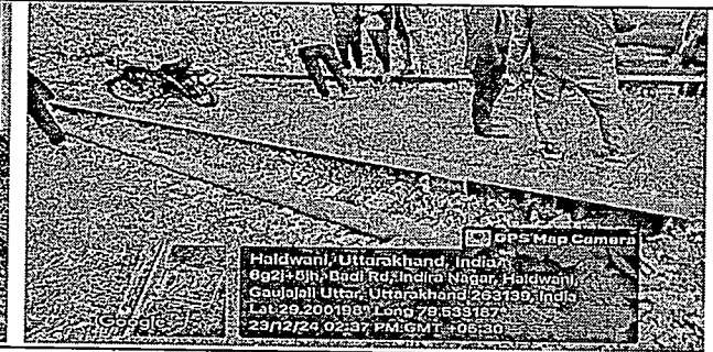
Photo 10: Weighing bridge not working at trenching ground
